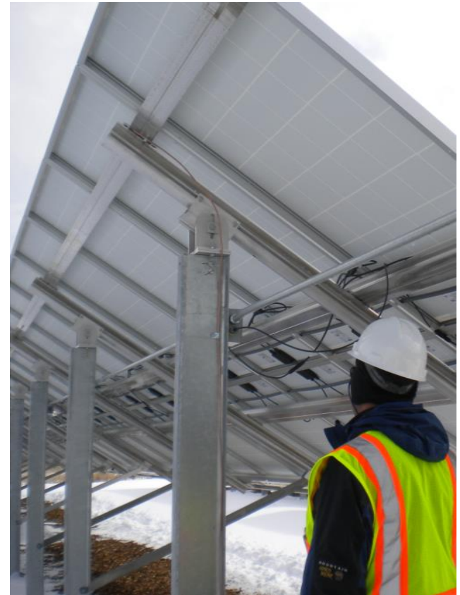
Inspection of a 67-kW PV system at Mesa Verde National Park. Photo by Andy Walker, NREL
