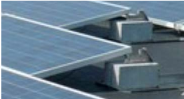
Photo by Mercury Solar Solution images.NREL.gov #18062
